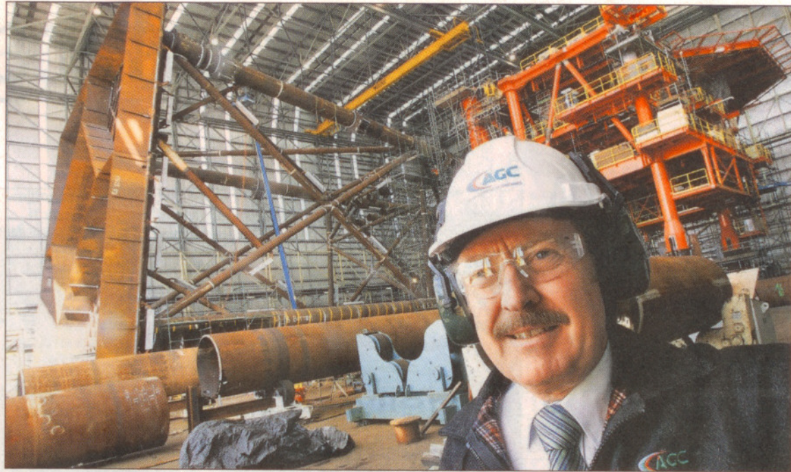
Big job: Mark Sawyer with the Blacktip gas production platform being built at Henderson. Picture: John Mokrzycki
